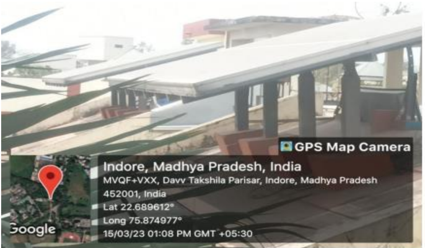
Solar Installation at School of Energy and Environment Studies
