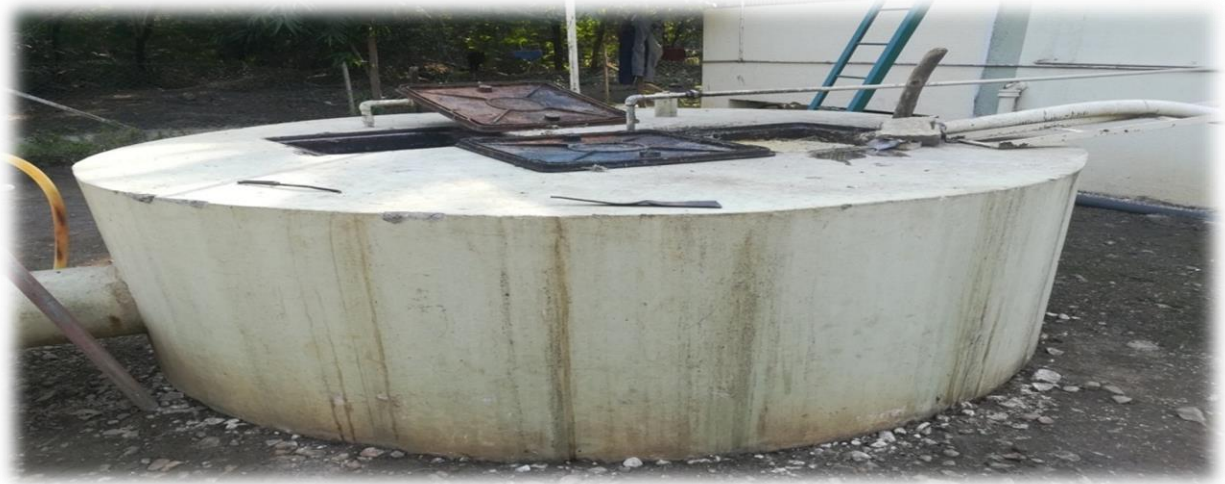
Picture 10: Pre-digester Tank (Two Chambers)
